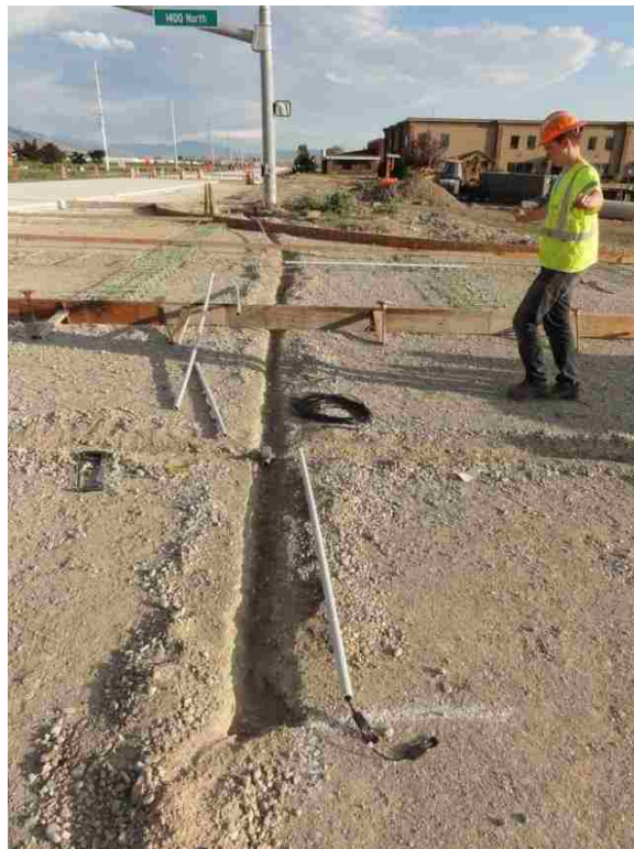
Figure 3-5: Sensor cables in PVC pipe.
