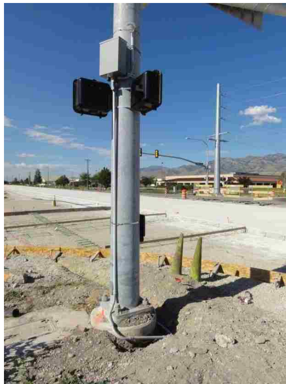
Figure 3-6: Utility box mounted on signal pole.
